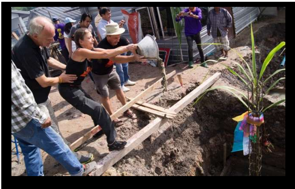
John and volunteer site manager Paul ensure Gill does not follow the concrete into the foundations during the traditional Buddhist ceremony to ensure the new hospital building is a success.
